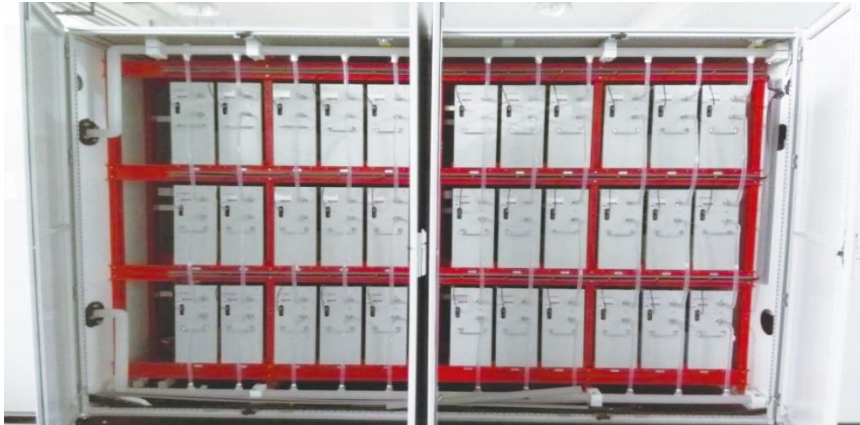
Figure 4.7 The layout of the units in the water-cooling power cabinet
