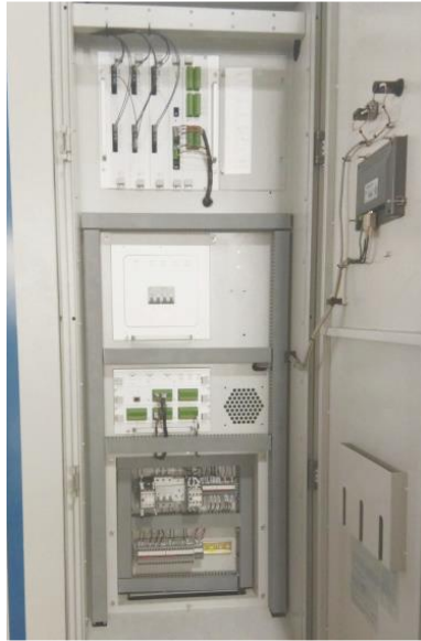
Figure 4.13 FDSVG control cabinet (for reference only)
