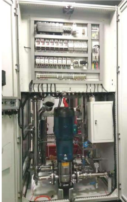
Figure 4.19 Water cooling control cabinet (for reference only)
